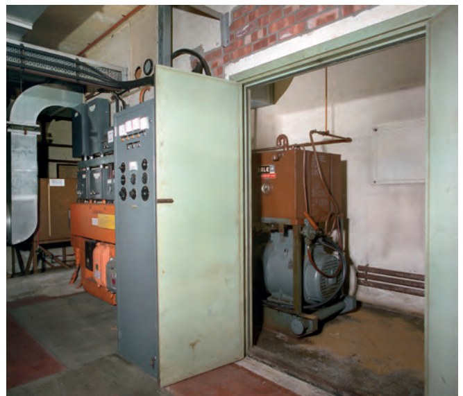
Standby diesel power plant in the original war room. Photo Nick Catford
